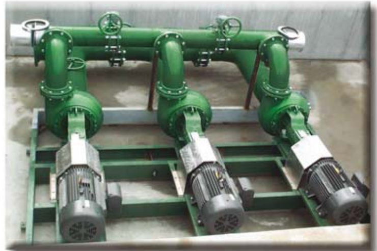
GreenLine 10X8X14 Flush pumps for 24,000 cow dairy with back-up pump.
